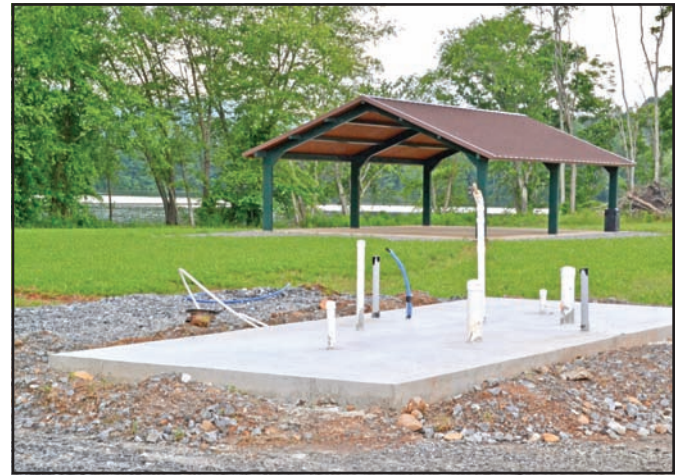
The new restrooms before walls and fixtures went up in Hiwassee Mayors Park. Photo by Mark Novak
