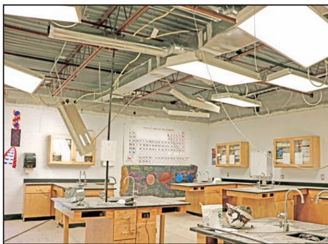
An interior view of a Towns County Schools classroom waiting for the installation of a new drop ceiling. Photo by Mark Smith
